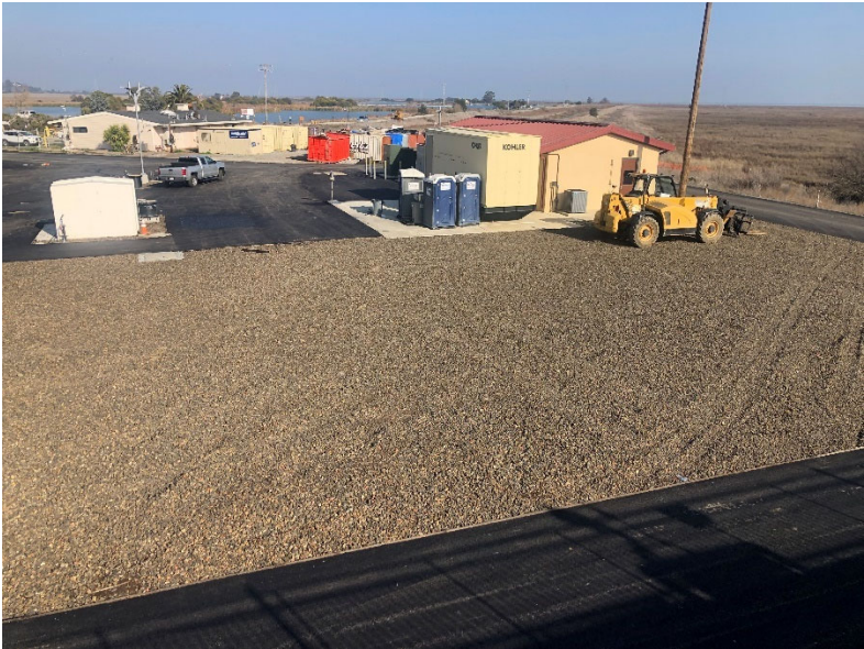
New Electrical Building
