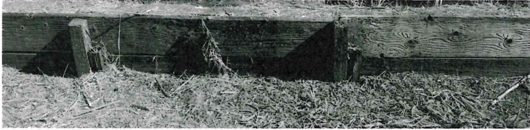
The Santa Venetia berm stands between homes and water in the South Fork Gallinas Creek.
