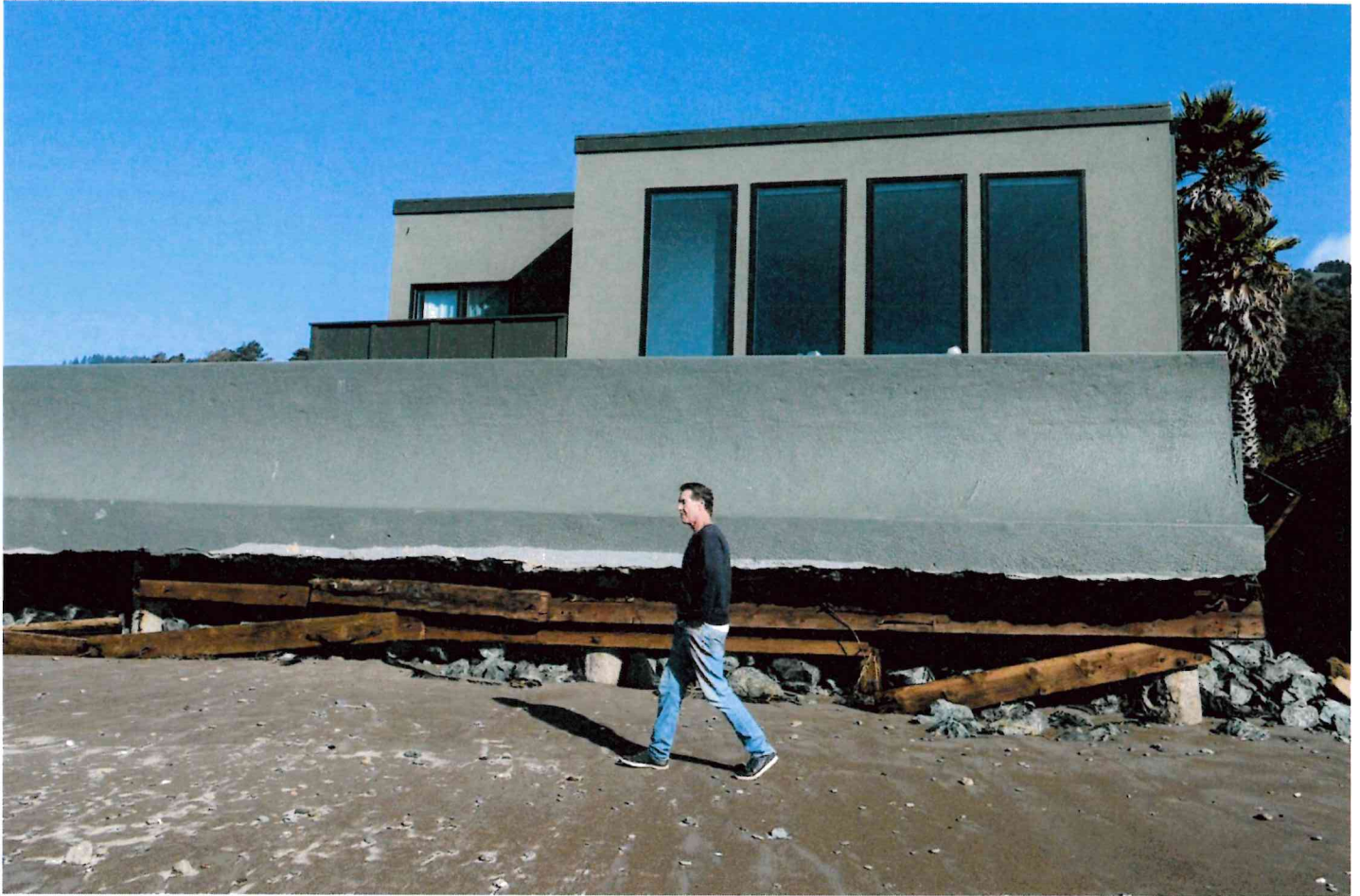
Kevin Loughlin of Petaluma walks by a storm-damaged home in Stinson Beach on Jan. 17, 2023. Stinson Beach was one of the key focus areas viewed as especially vulnerable to the effects of flooding from rising water. ALAN DEP — MARIN INDEPENDENT JOURNAL
