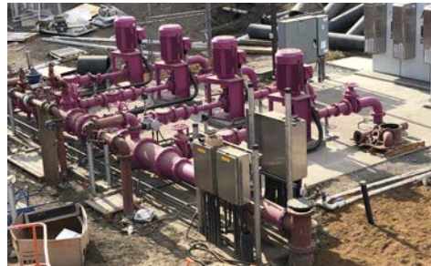
Recycled Water Distribution Pump Station
