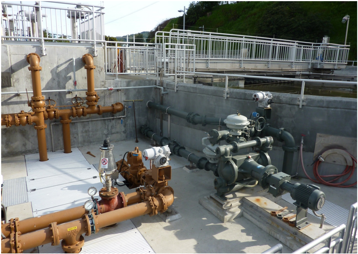
Primary clarifier sludge pump facilities
