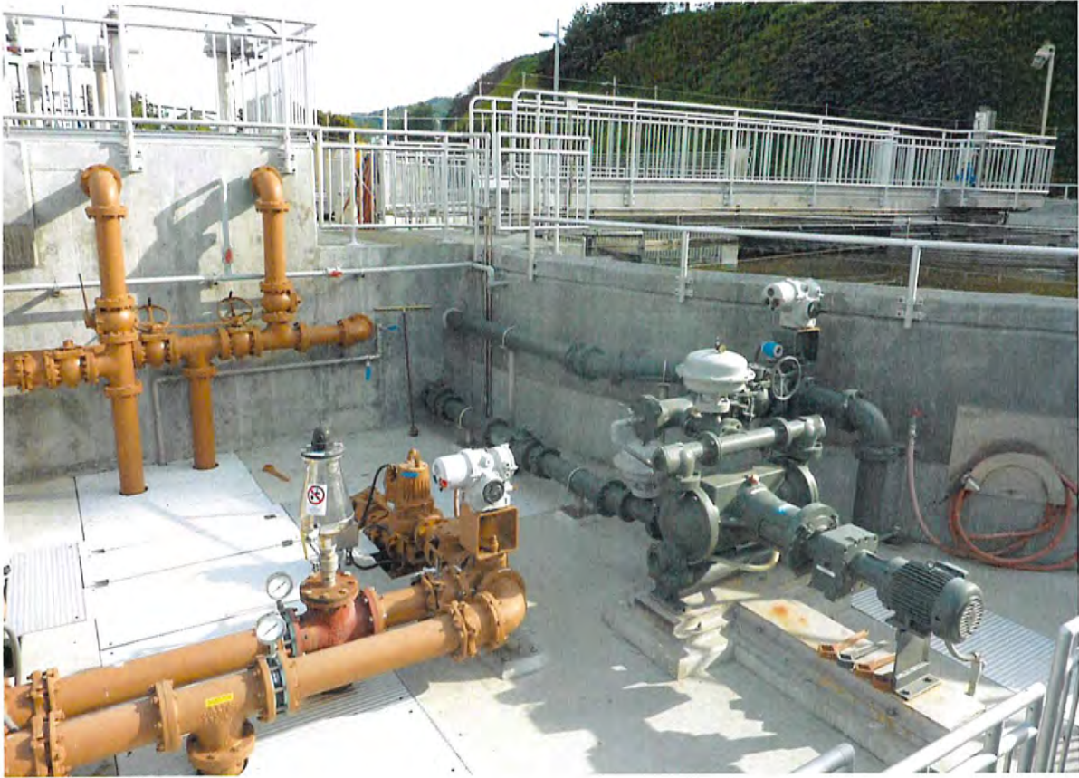
Primary clarifier sludge pump facilities
