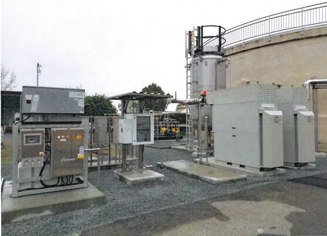
Biogas Recovery System Microturbines
