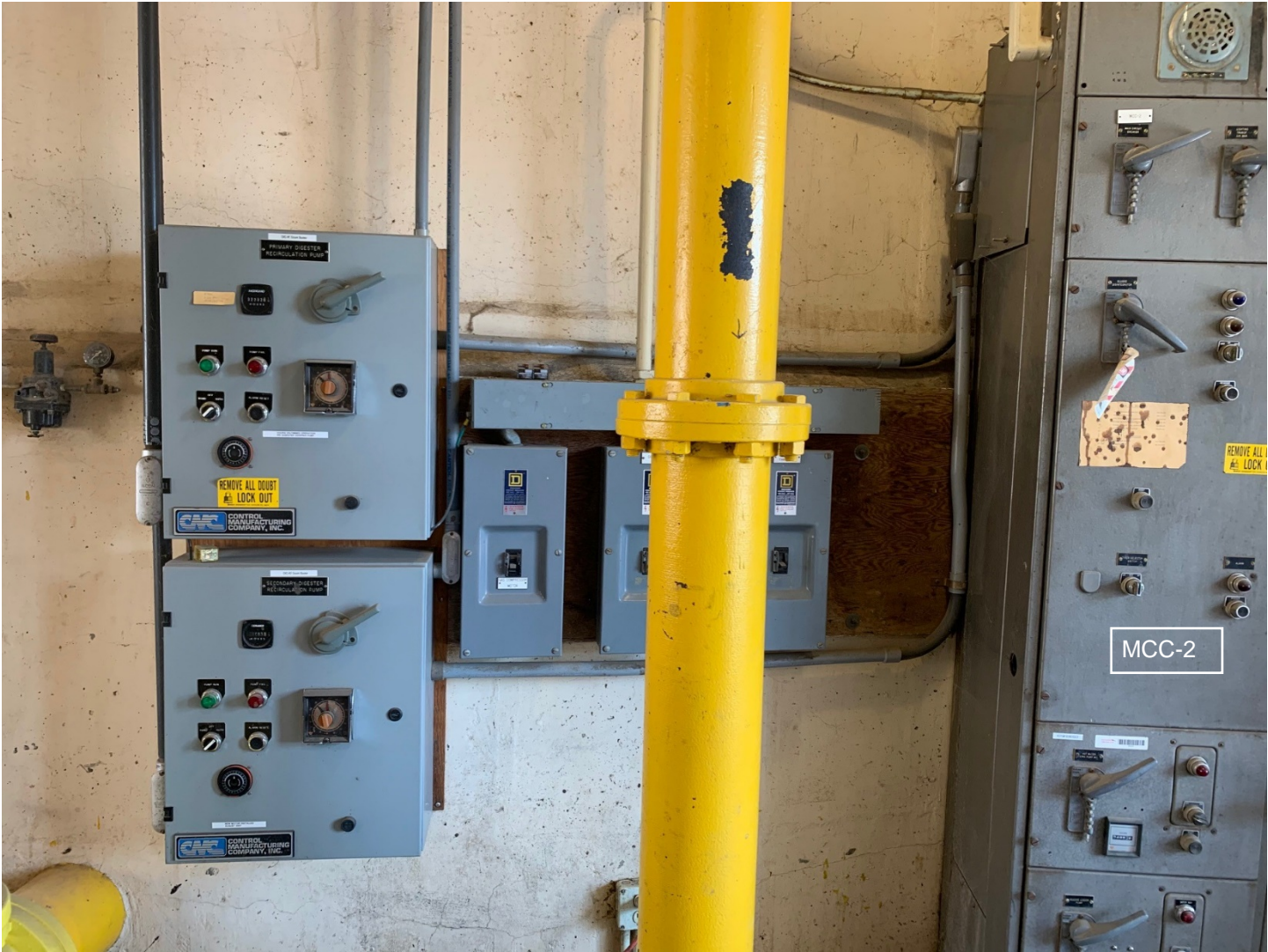
Figure 4. Existing control panels for “scum buster” pumps.
