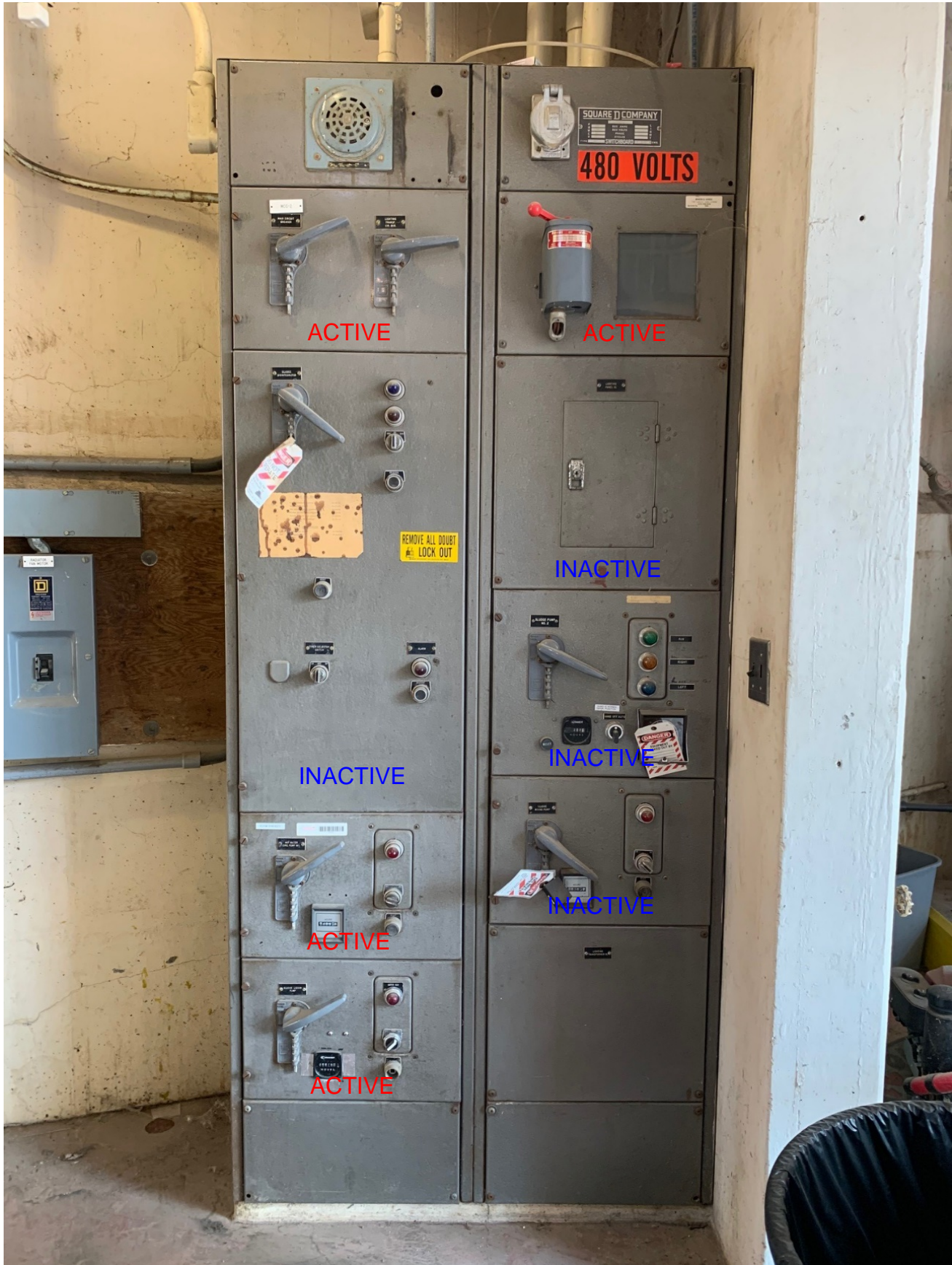
Figure 3. Existing MCC-2 in Digester Room.
