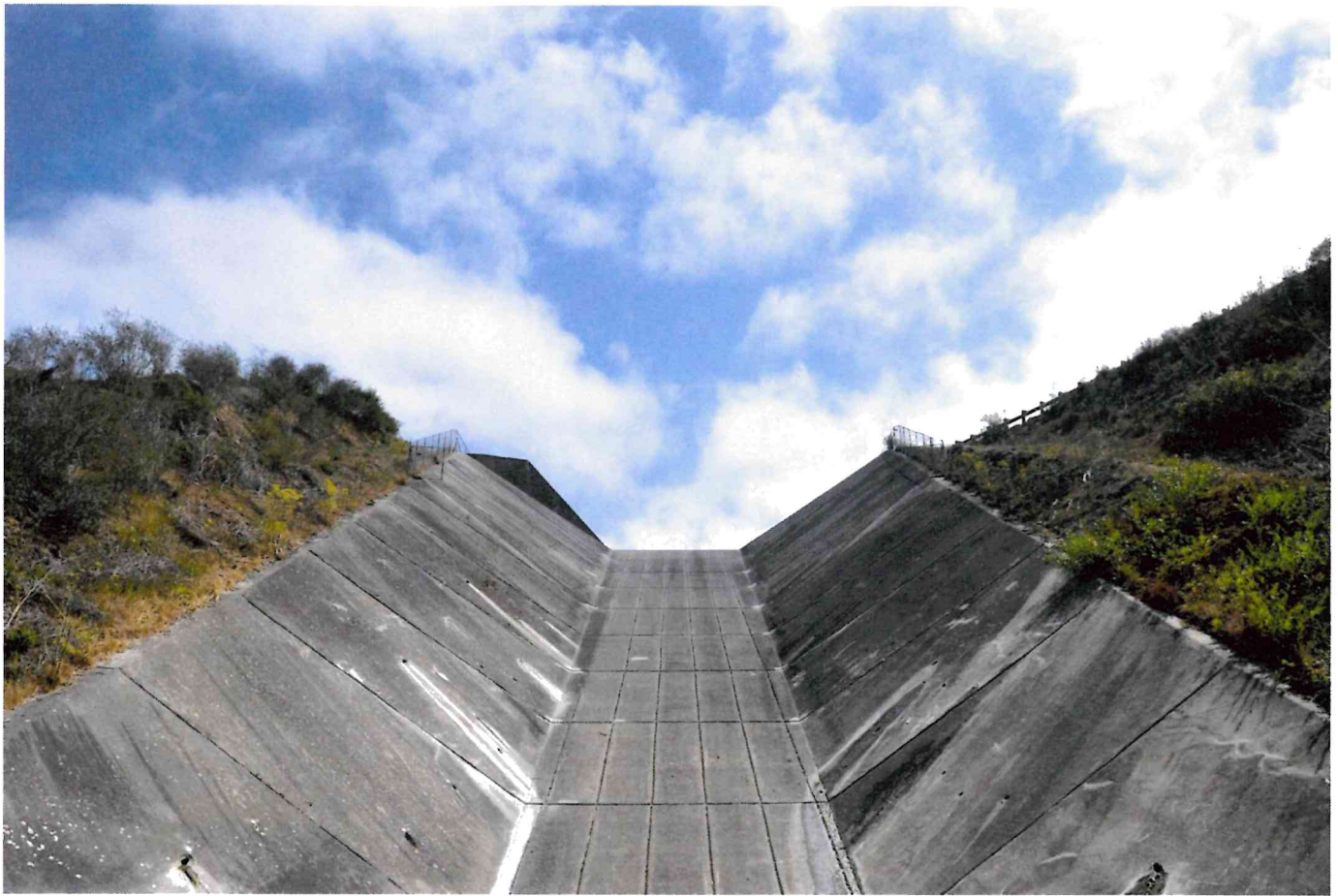
The spillway of SoulaJule Reservoir in western Marin. The Marin Municipal Water District plans to repair spillways at various dams. ALAN DEP — MARIN INDEPENDENT JOURNAL
