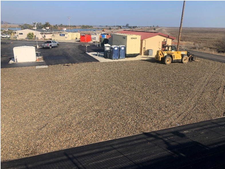
New Electrical Building
