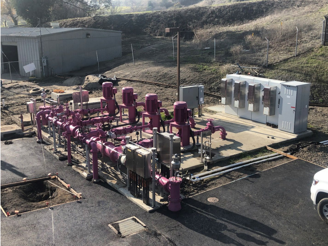
Distribution pump facilities
