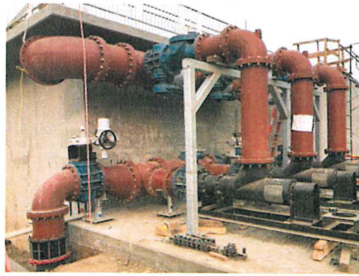
New Internal Recycle Pump Station
