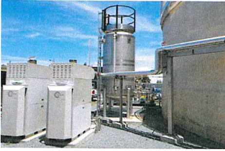
Methane Gas Powered Microturbines
