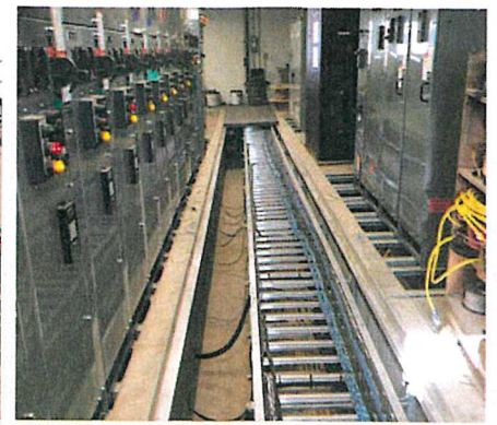
New Electrical Building Equipment and Cable Trays
