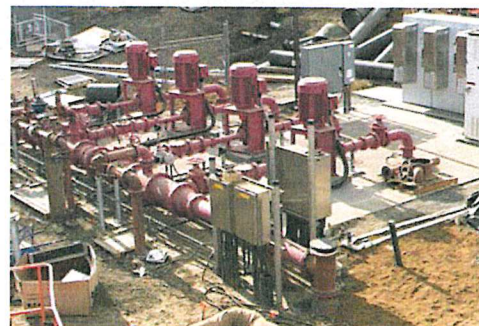
New Recycled Water Distribution Pump Station
