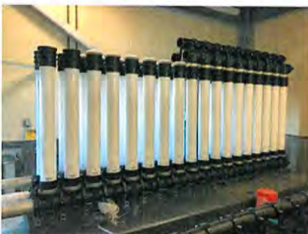
New membrane filters in the Recycled Water Treatment Facility.
