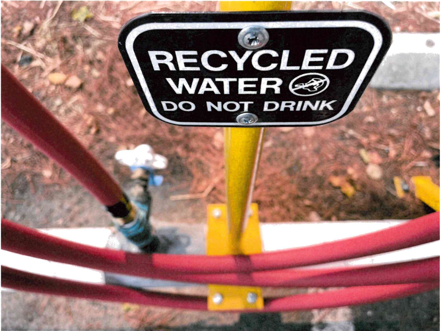
A recycled water filling station stands at the Marin County Civic Center in San Rafael in 2021.
