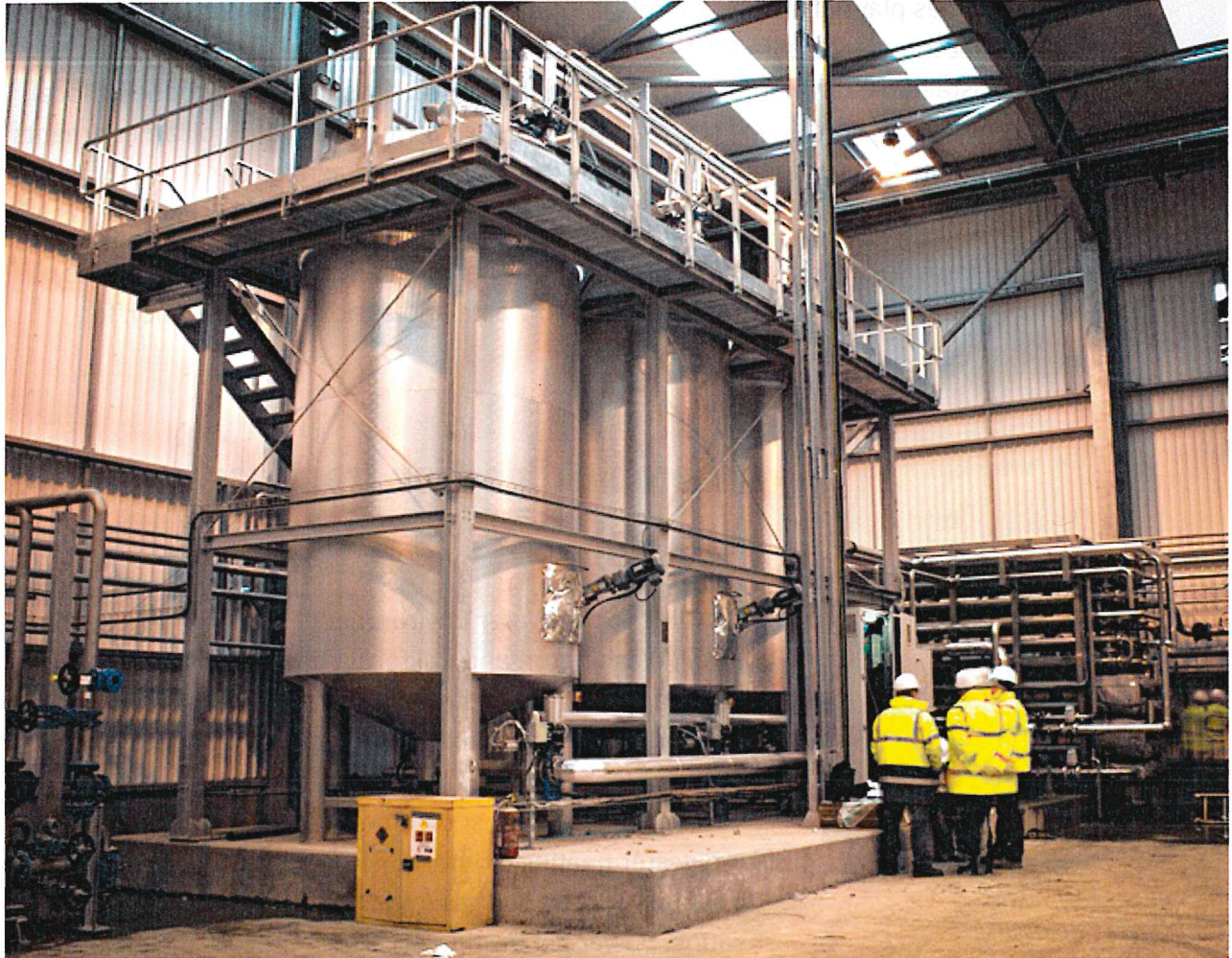
HRS sludge pasteurization tanks
