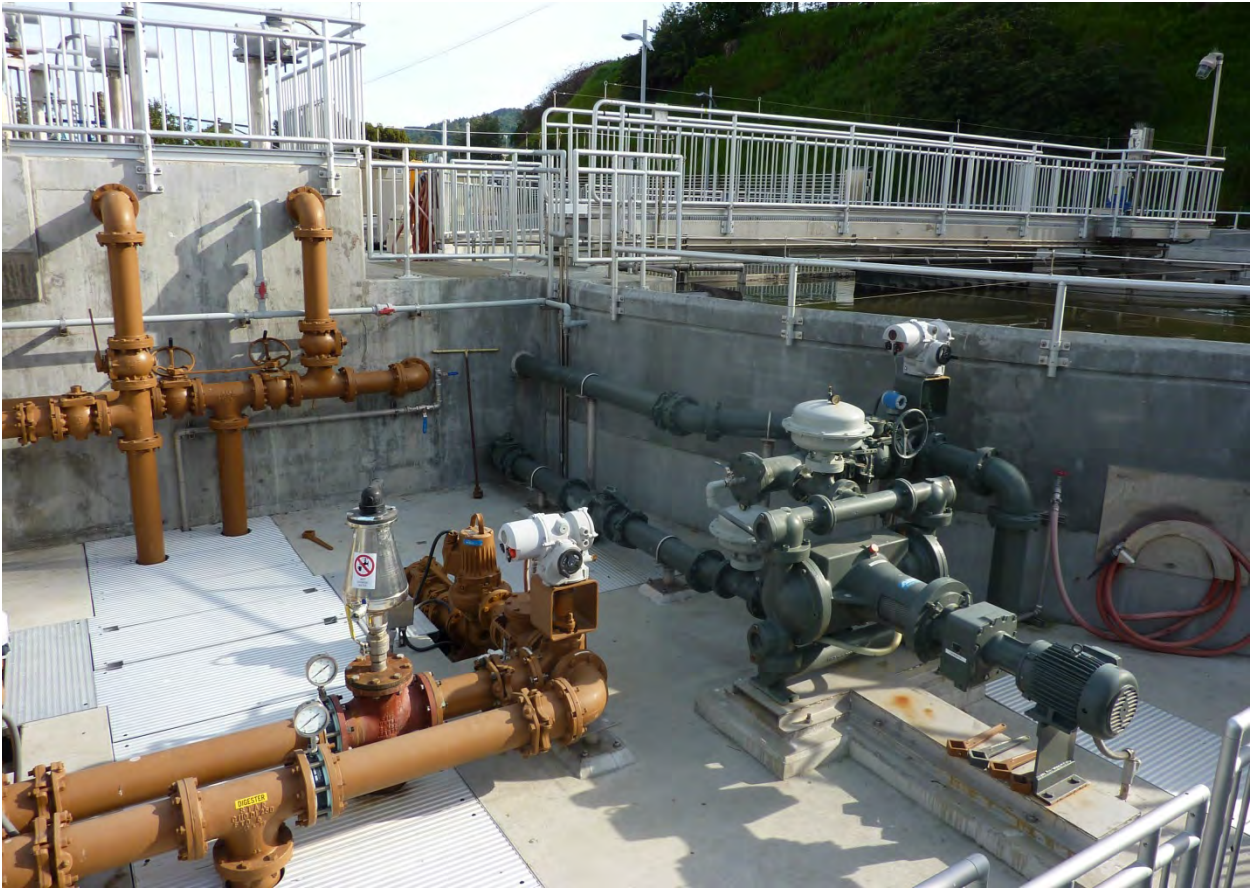
Primary clarifier sludge pump facilities
